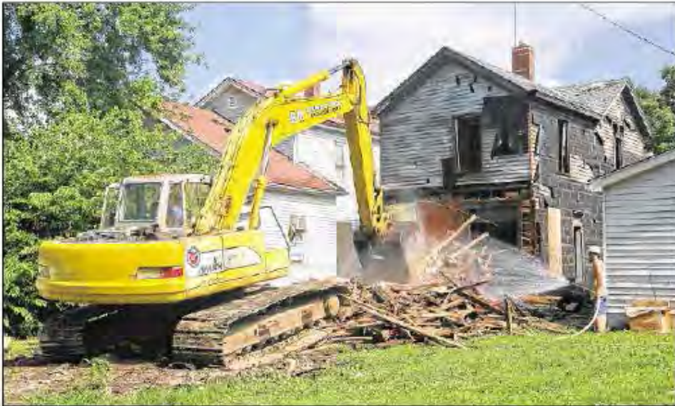
Demolition crews tear down a house at 335 Hanover St. on Friday. The state and federal governments have just awarded Butler County an additional $1.8 million in Hardest Hit funds to continue purging dilapidated properties. GREG LYNCH/ STAFF
